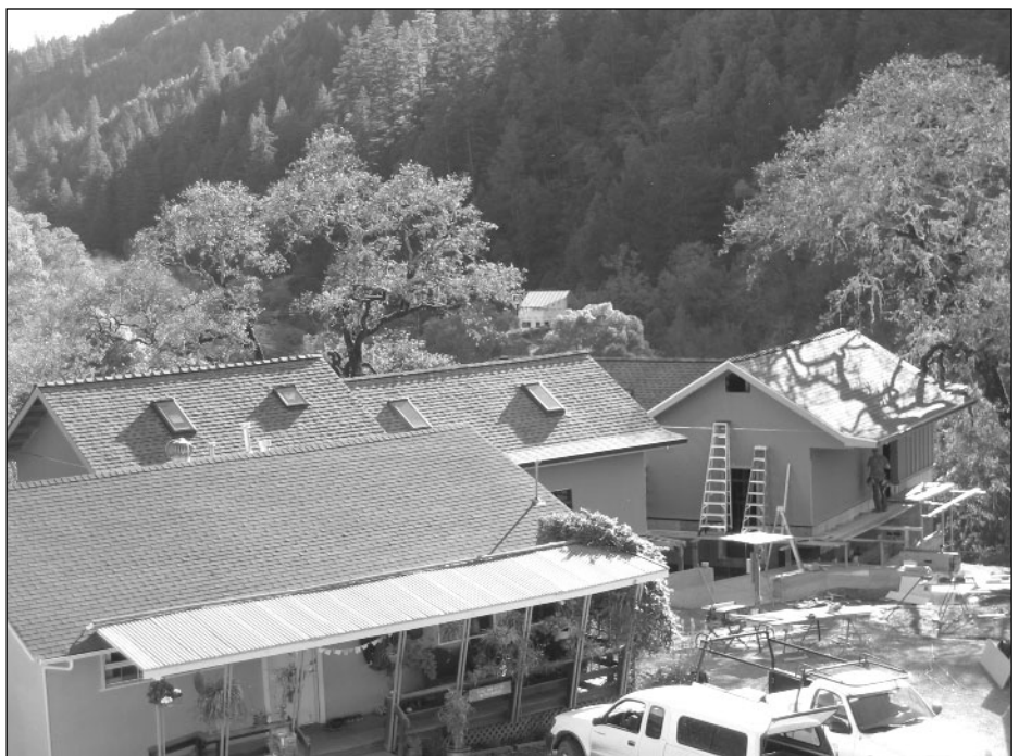
New cloister office building (back left) and restrooms (back right) under construction
